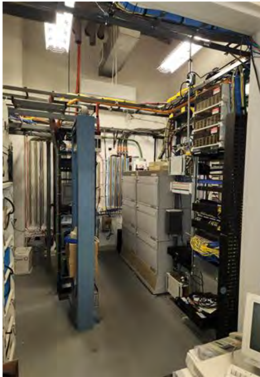
SERS Telecom Room
